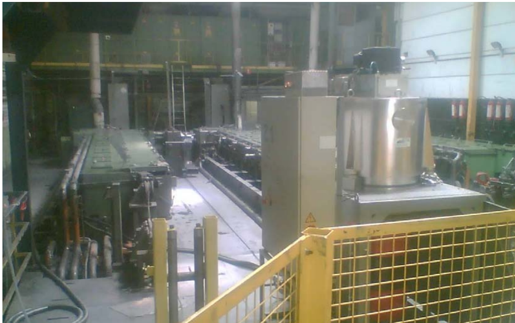
Picture #3: The STA centrifugal separator, connected to 3 wire drawing machines.
