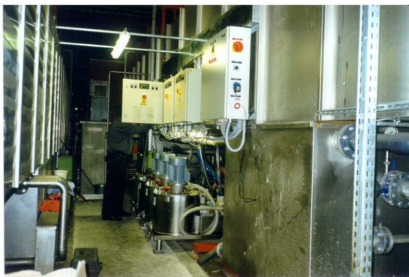
4 S-15 centrifugal separators installed at active zones 1 and 2
